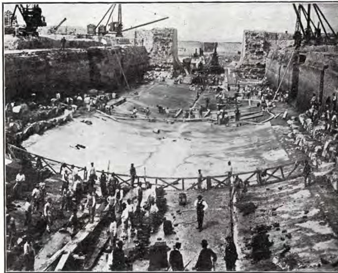
Here are shown the walls of the Pampean formation and alluvium still exposed after the concrete floor had been laid, with the sump and pumping machinery as in the view above.
